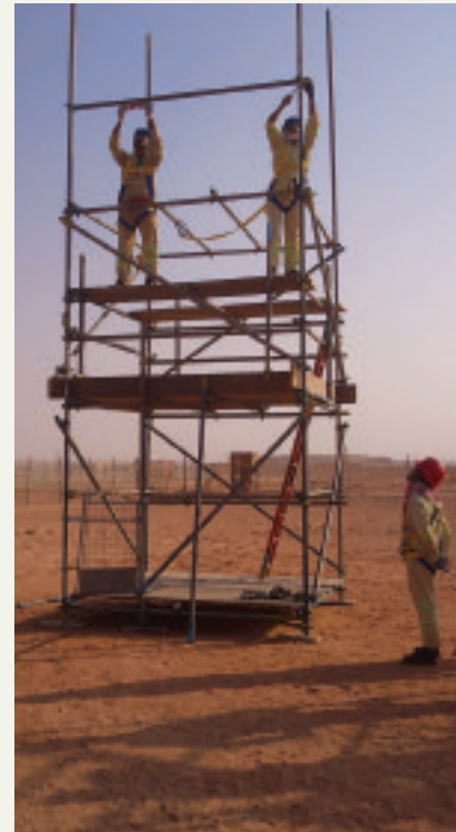
TG20:13 is likely to have a positive impact on scaffolding operations across the globe. Here Simian Risk carries out work in the Middle East
